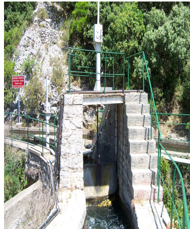
Figure 2: Partiteur Right Bank regulation gate
